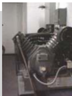
Air Compressor – Full Visible
